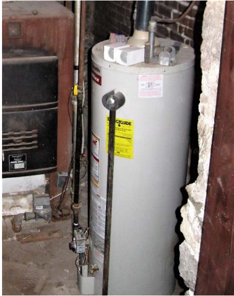
Figure 63: Existing 30-gallon gas-fired water heater provides all domestic hot water supply in the building
