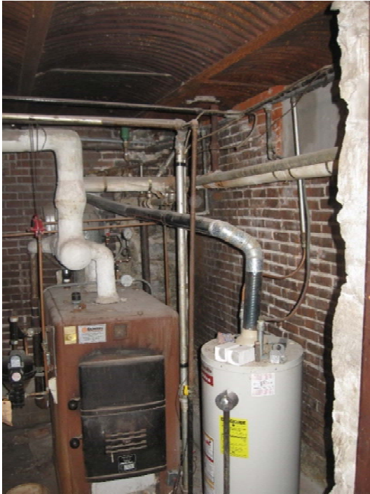
Figure 56 Basement Mechanical Room/boiler
