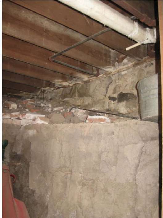
Figure 57 Crawl Space/crumbling foundation/rotted sill
