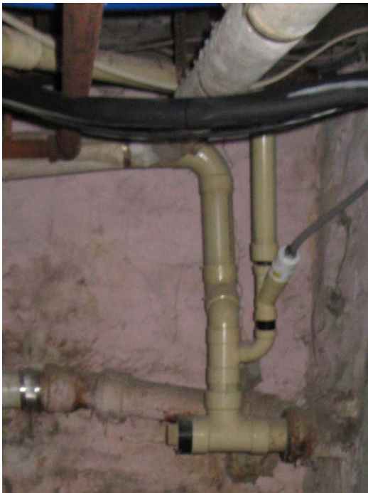
Figure 59: Cast Iron and PVC Piping Comprising 4" Building Drain Leaving the Basement on the North
