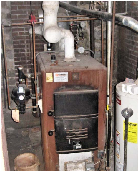
Figure 65: Existing Low Pressure Steam Boiler Designated to Serve in Standby Capacity
