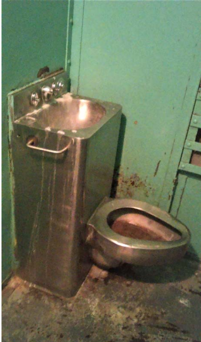
Figure 62: Rust and mineral deposits form on security plumbing fixture in east cell
