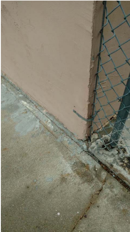
Figure 44 Un-flashed building corner
