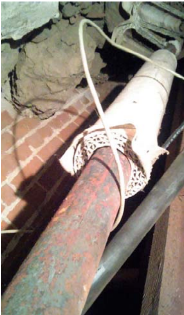
Figure 66: One of a multitude of friable asbestos conditions
