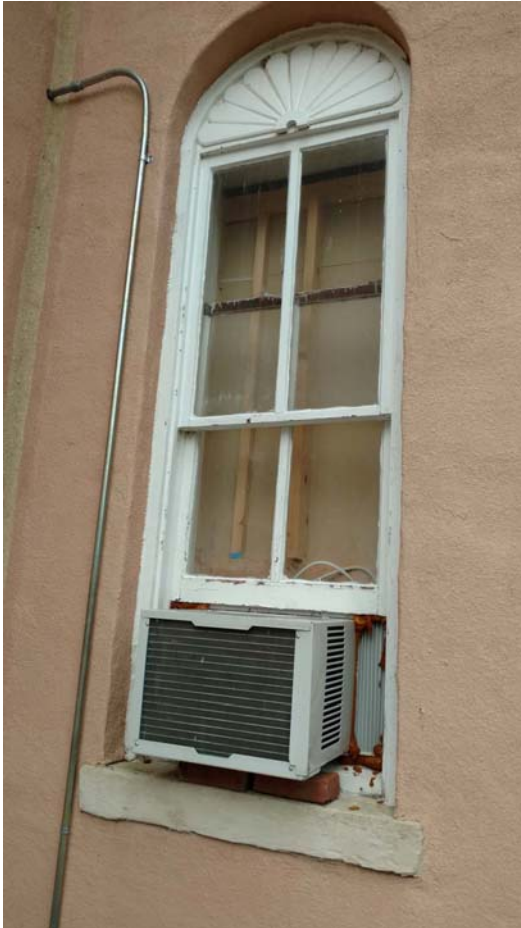
Figure 40 Typical window with interior furring The sunburst or fan molding at the head is likely evidence of a true brick arched lintel
