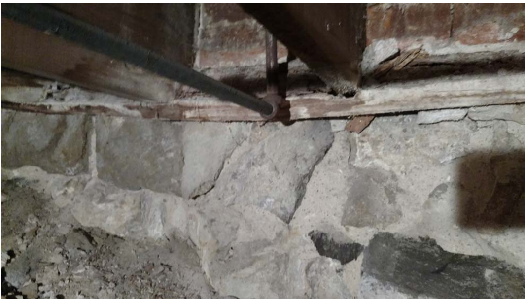
Figure 58 Exposed limestone foundation in crawl space, and damaged floor joist sill plate
