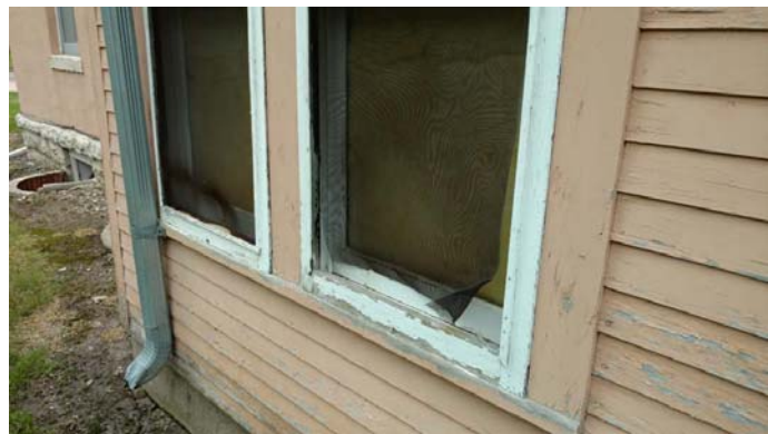
Figure 43 Torn screen and single-pane glass into the Pantry addition. The interior Pantry area has been walled off.
